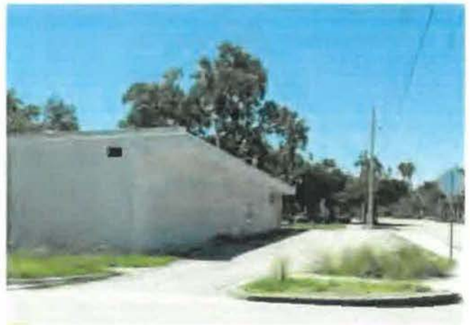
All windows and doors boarded.
